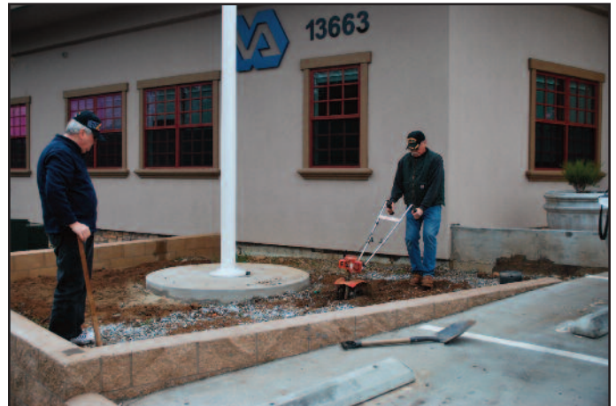
Frank Smart and Bob Walker level the ground where the bricks will be placed. Gereon Rios has begun assembling the Memorial.
